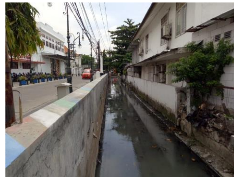
Figure 4. The sewer problem drains into the old city drainage system.
