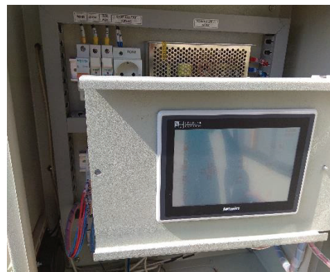
FIGURE 4. Inside view of the control panel, along with touchscreen LED
