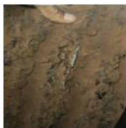
Figure 1: Slagging In Boiler
