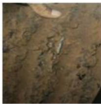
Figure 1: Slagging In Boiler
