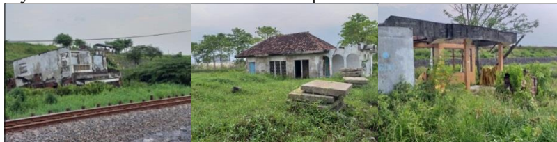
Figure 4. Several houses in the area impacted by the mud disaster Lapindo which were damaged and left behind by residents. (Source: Author Documentation, March 19, 2019)
