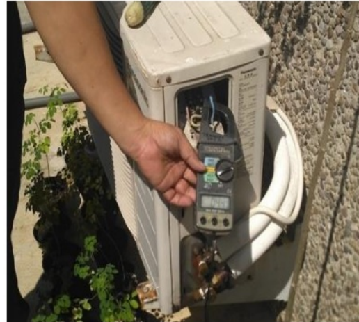
Figure 2: Electrical current measurement
