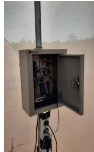
Fig. 2. The installed smart device for environmental engineering
