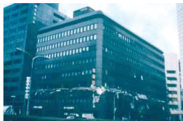
FIGURE 4. The Kobe Earthquake of 1995, the third story of the commercial building was lost and the above stories fell on it (source: Bachmann 2003).
