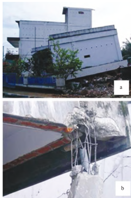
FIGURE 10. Bengkulu Earthquake in 2007, a). The collapsed shophouses, b). Planting utility pipes in the column (source: Boen 2007a).
