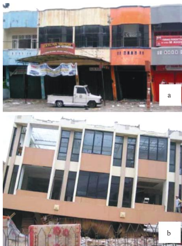
FIGURE 9. West Sumatra Earthquake in 2009, a). Ruko/ shophouses undergoing residual drift, b). The first floor of the shophouses collapsed (source: Wilkinson et al. 2012).
